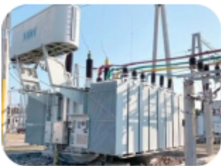
Energy consumption management
