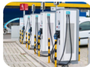
Charging and battery-swapping stations
